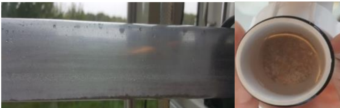
Figure 17 Residual egg shells in the wall pipe and siphon.
